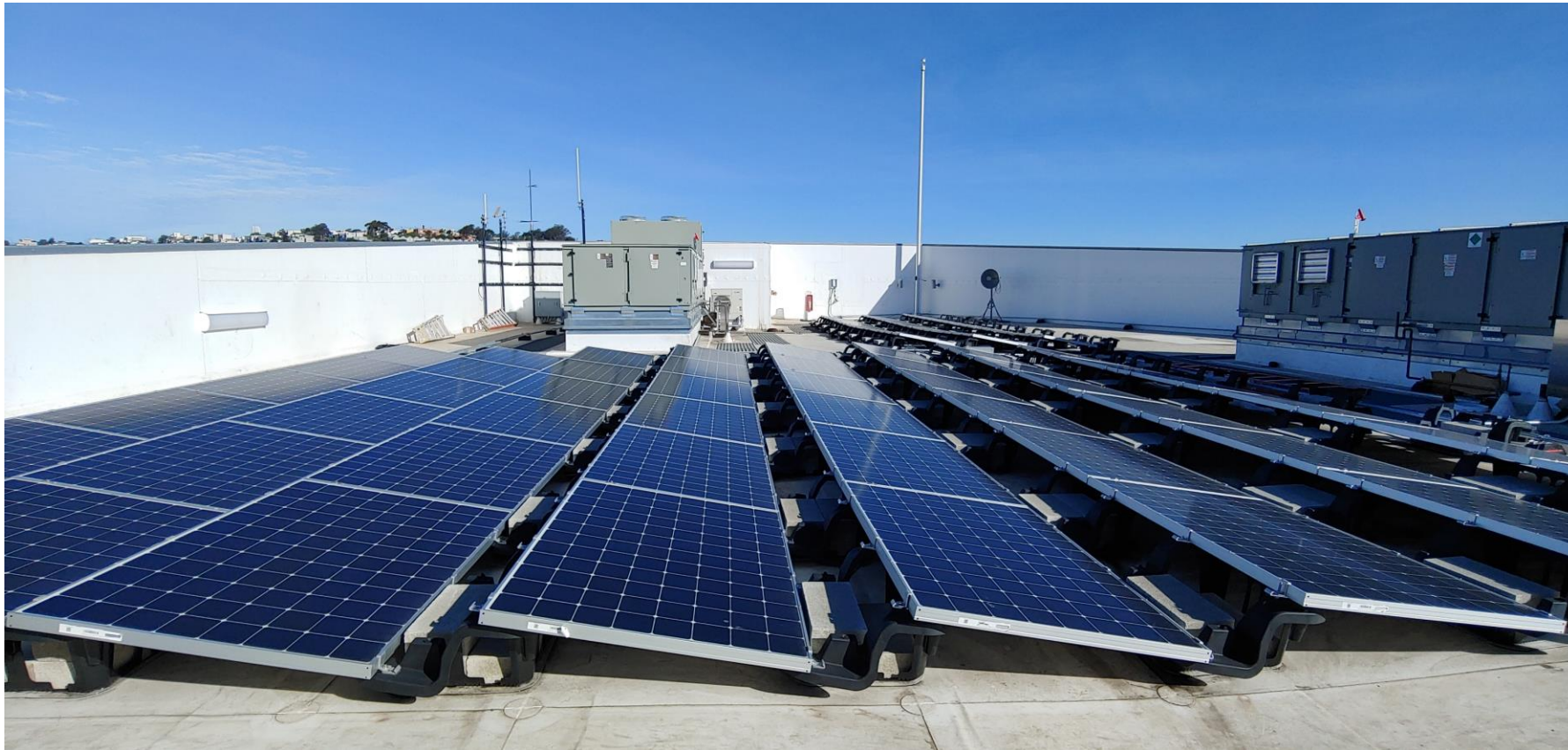
Solar Panels on Roof
