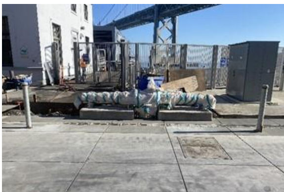
Concrete Base at EFWS Fireboat Manifold
