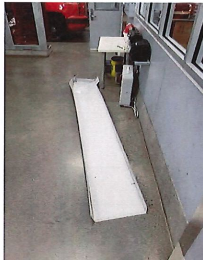
Piece of flashing that had blown off
