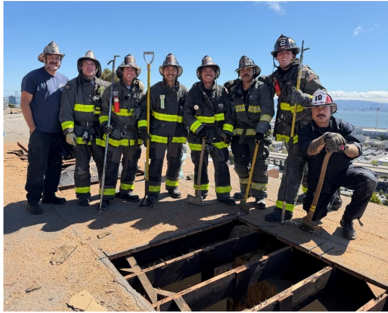
Truck 2 on the roof after opening the hole with saws and axes. (Instructors Lt. Sean McCarthy and Lt. Figueroa)
